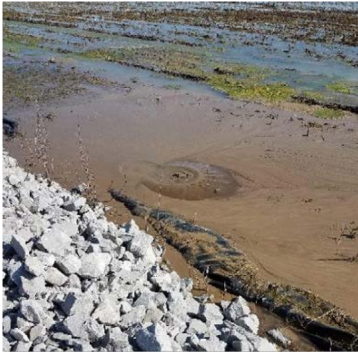
Image of sand boil (underseepage), from 2019 flooding, courtesy of USACE.
