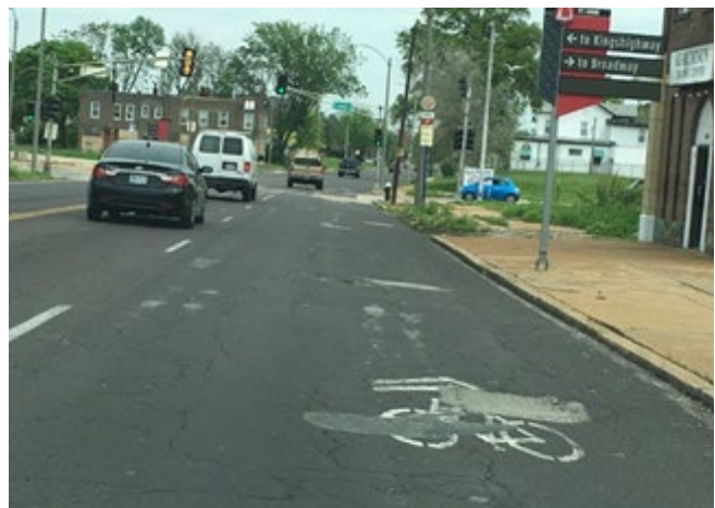
Poor pavement condition and patching over shared lane markings on North Grand Avenue.
