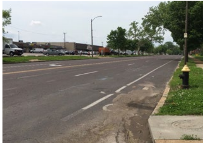
Debris covering bike lane and marking on South Broadway, with faded shared lane marking visible in the outside travel lane.
