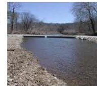
Fish-friendly low water crossing
